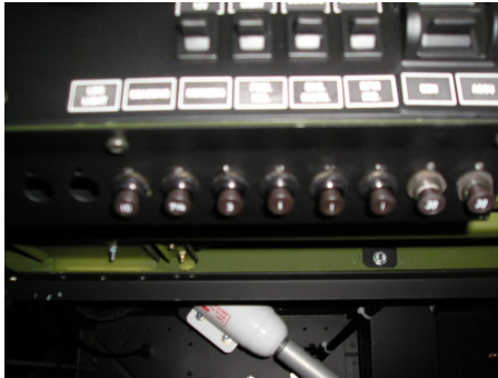
Picture: Circuit breakers under the instrument panel
